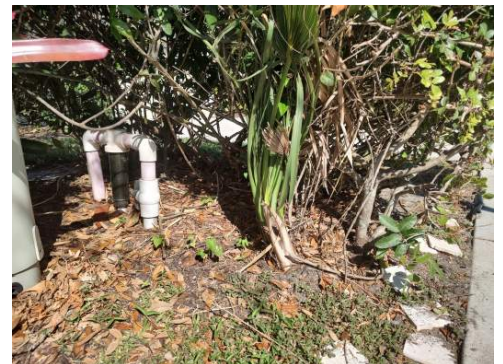
Example of overgrown valve cover
